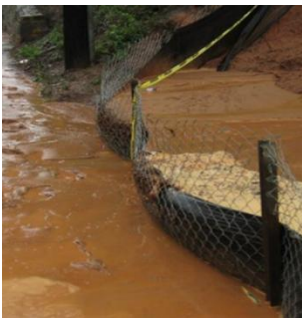
Construction Site Runoff
