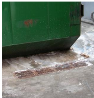
Dumpster Compactor Leaks
