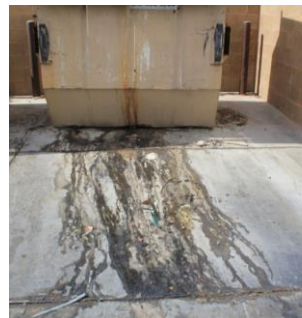
Grease Container Leaks
